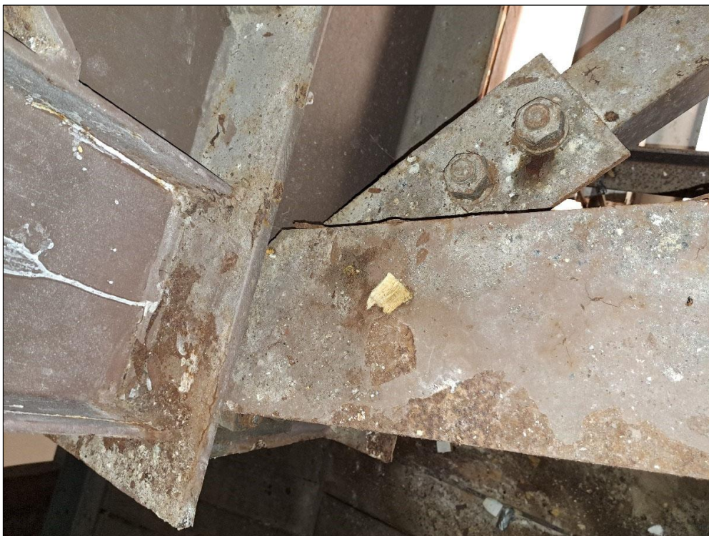
Figure 25 NE corner bottom connection.
