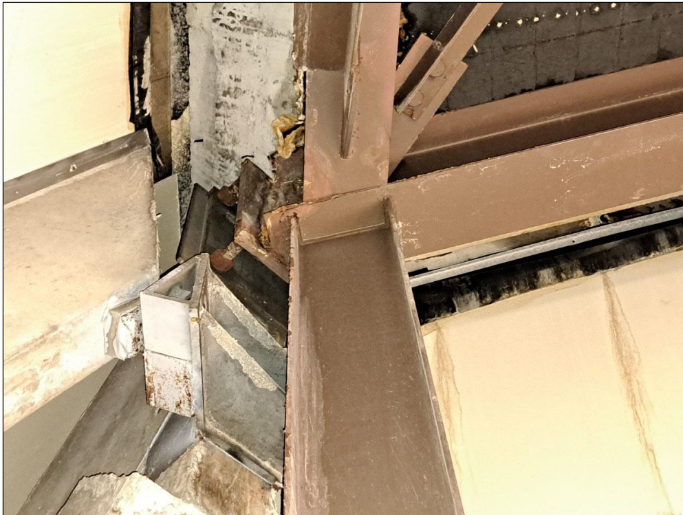
Figure 26 NE corner bottom connection.
