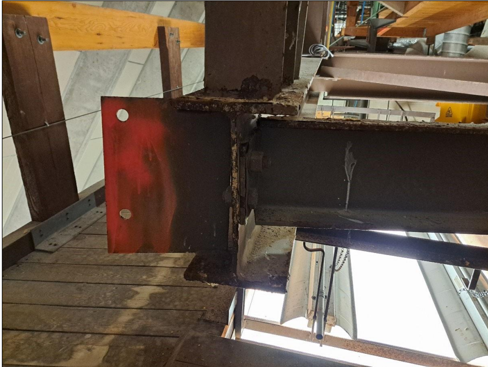
Figure 24 NE corner bottom connection.
