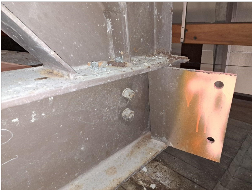
Figure 23 NE corner bottom connection.
