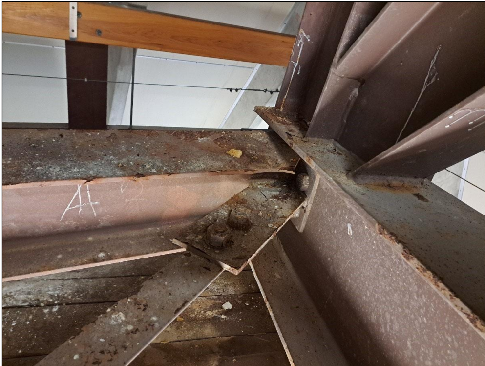
Figure 22 NE corner bottom connection.
