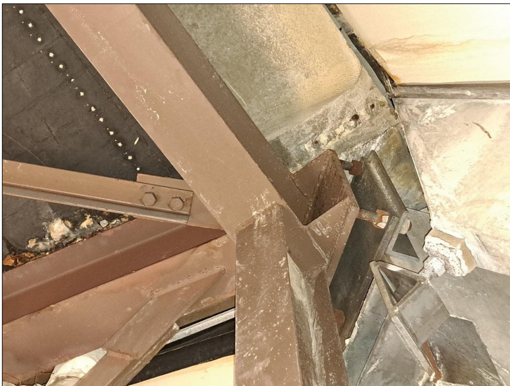
Figure 27 NE corner bottom connection.
